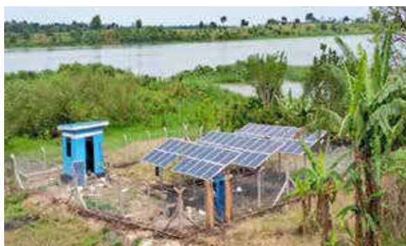
Photo 8- 5: Namutya Small Scale Irrigation Scheme in Kayunga District
