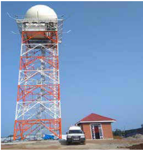
Photo 10- 35: First weather radar fully installed and operational in Kigungu
