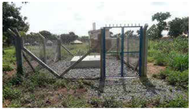
Photo 7- 3: Sludge Holding Tank in Nyumanzi
