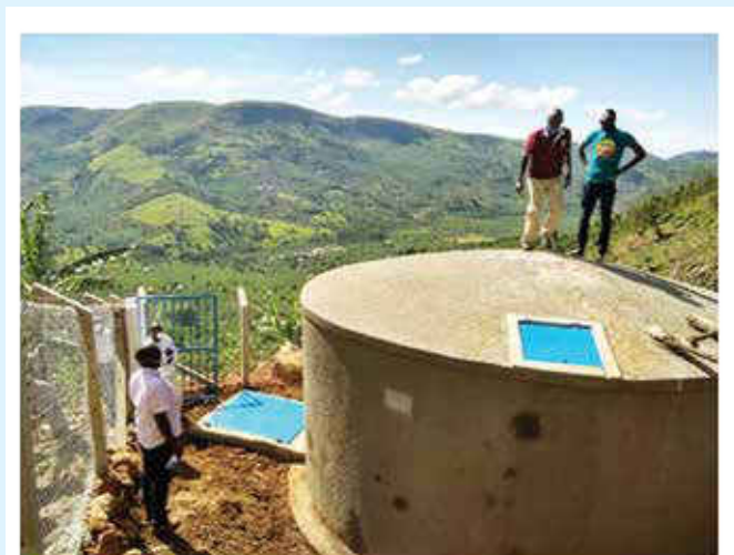
Photo12- 5: The 30,000 Litre reservoir tank - serves the upper line
