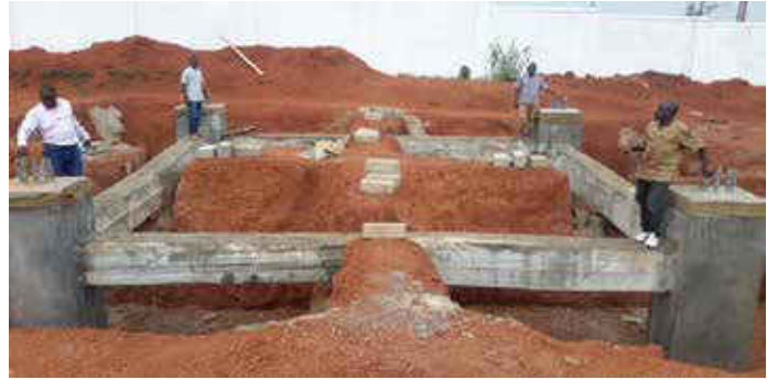
Photo 10- 36: Radar tower works for the second weather radar at Mwizi hill in Rwampara
