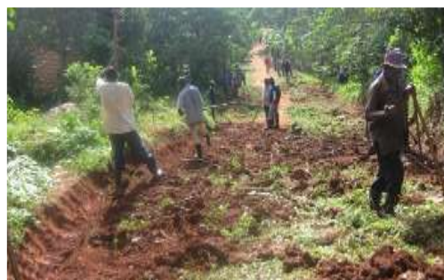
Figure 5: Kikandwa community members applying the road water harvesting technique/innovation to sustain and maintain the road. Photo by KEA.
