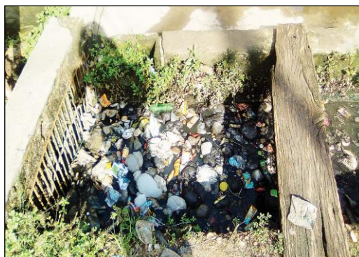
Figure 2: Indiscriminate waste disposal in drainage channel in Kiroombe Village, Makindye 1 Parish, Makindye Division, Kampala. Photo by Environmental Alert.
