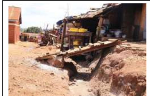
Figure 1: A restaurant in Mbuya II located at the drainage channel before construction. Photo by Environmental Alert.
