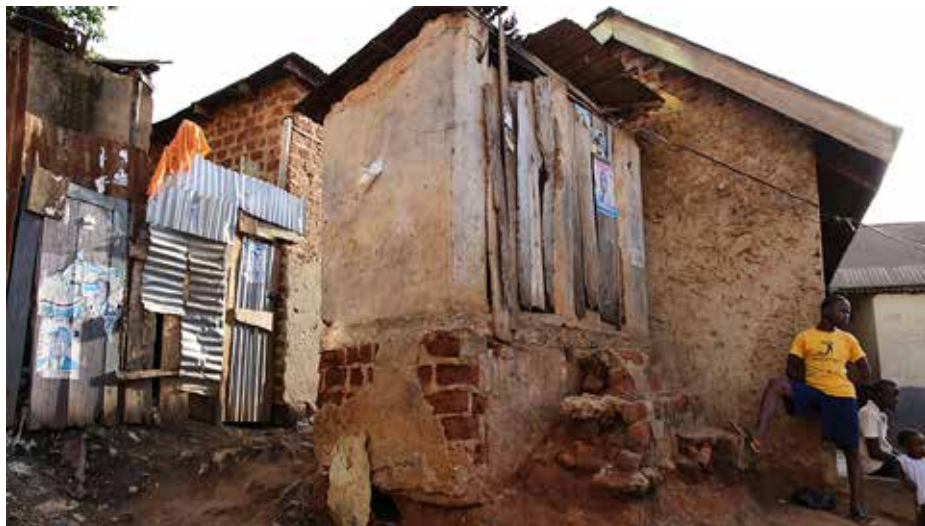
Figure 8: Dilapidated household toilet unit in Mengo ward, Kampala Central Division.
