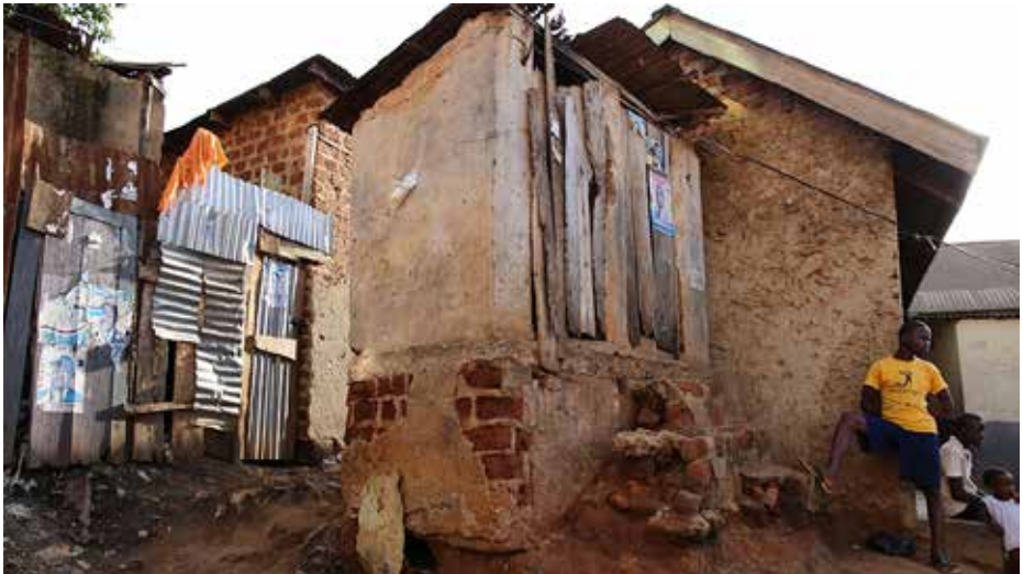
Figure 8: Dilapidated household toilet unit in Mengo ward, Kampala Central Division.
